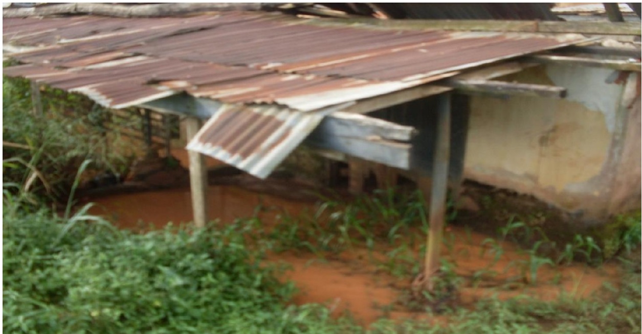
Figure 10. Abandoned residential house in flood area.
