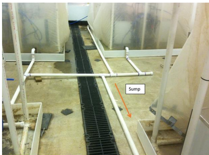
Figure 11: Gravity-flow spent coolant return network on swine calorimetry experiment at the USDA Farm Animal Behavioral Laboratory (FABL) swine experimentation room.
