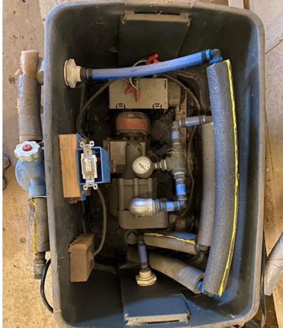
Figure 3: Next generation modular filtration and pressure supercharging system in once-through coolant supply installation at the Purdue Animal Science Research and Education Center (ASREC) swine farrowing barns.
