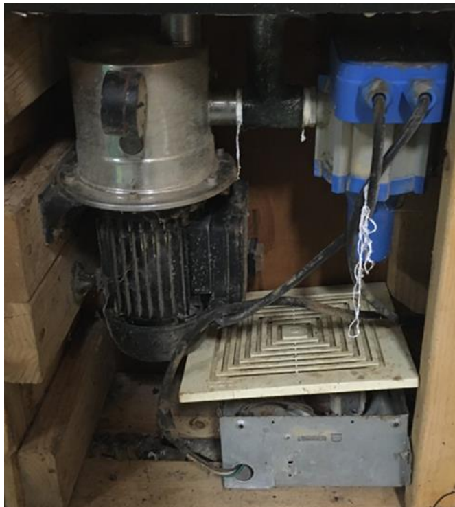
Figure 2: Initial filtration and pressure supercharging system used in once-through coolant supply installation at the Purdue Animal Science Research and Education Center (ASREC) swine farrowing barns.
