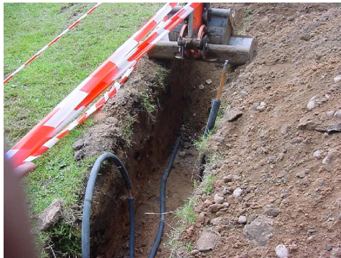
Figure 21. A photograph shows the earth loop vapour and liquid (Abdeen et al., 2009).
