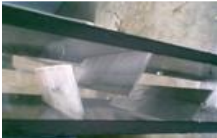
Figure 6. Baffles in rectangular duct.
