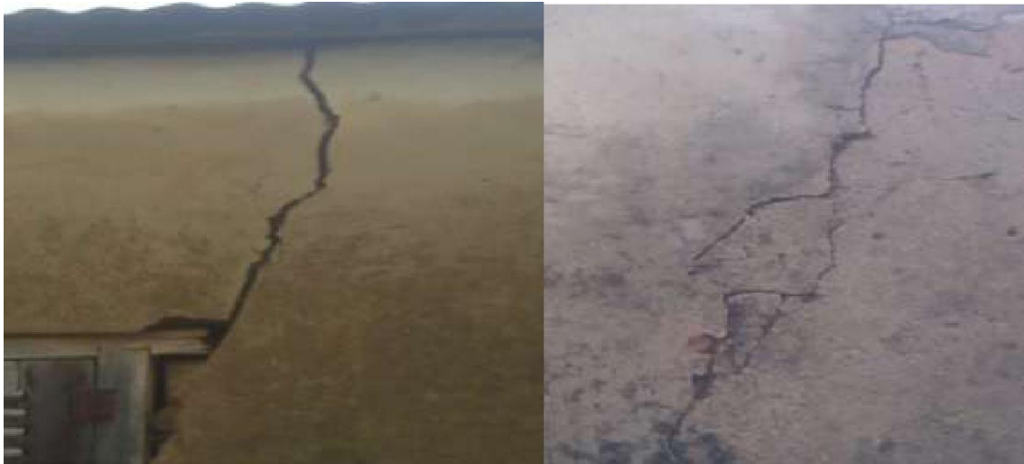
Figure 3. Cracks on the cement block wall.
