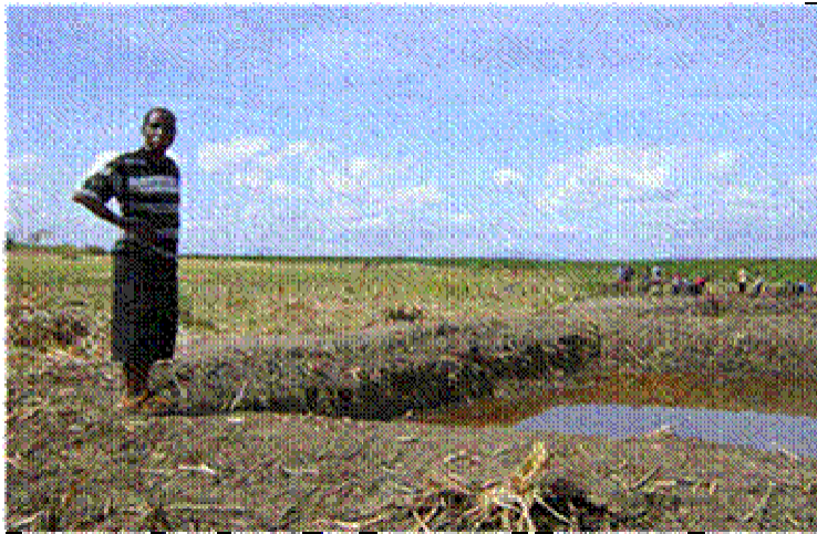
Figure 15. A member of the research team supervising ponds being constructed and compacted
