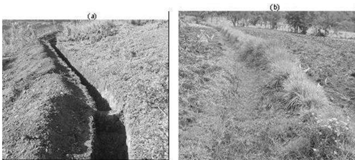
Figure 3. Typical level soil bunds in upper watershed; (a) newly constructed (b) 6 years old and planted with grass.
