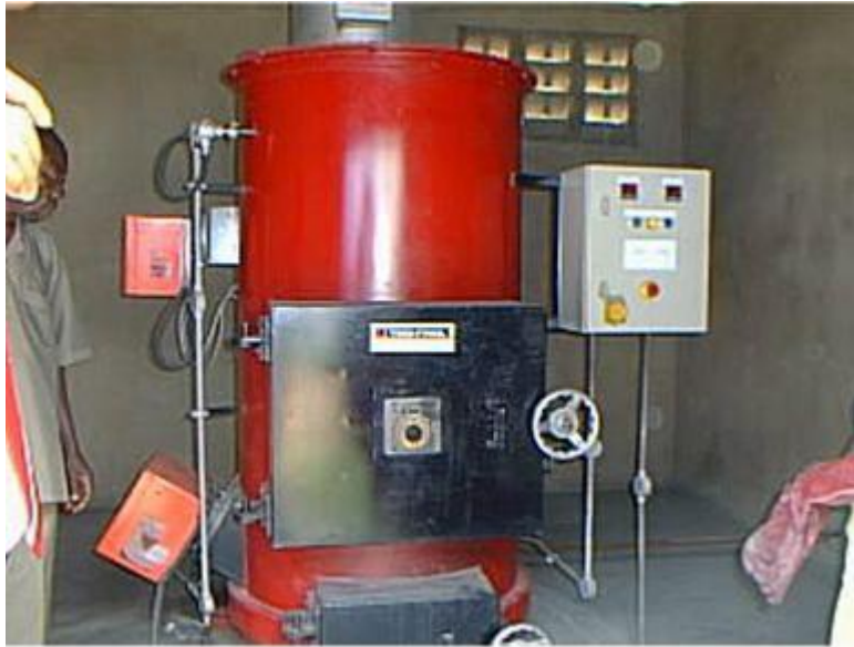
Plate 4. Over-utilized incinerator at UCH Ibadan.
